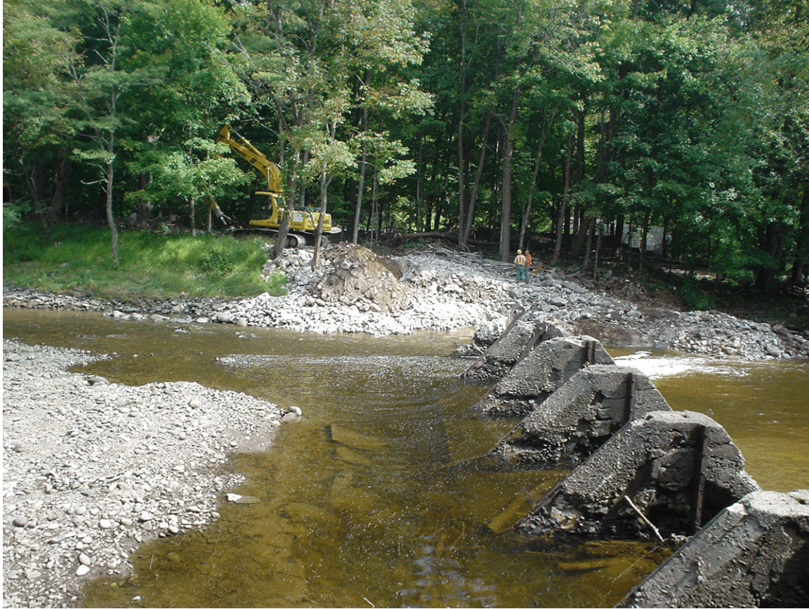
Appendix Figure 5. Neversink River and Cuddebackville Dam during dewatering period in September, 2004.
