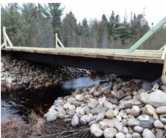
After: New bridge on the East Branch of the Two Hearted River. Courtesy of The Nature Conservancy/Emily Clegg
